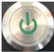
Fig. 11: Main battery switch not pressed
