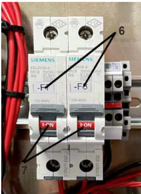
Fig. 21: F7 and F8 position "ON"
